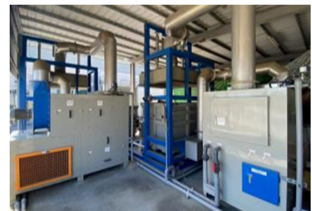
▲ Catcher's Sludge Drying System
